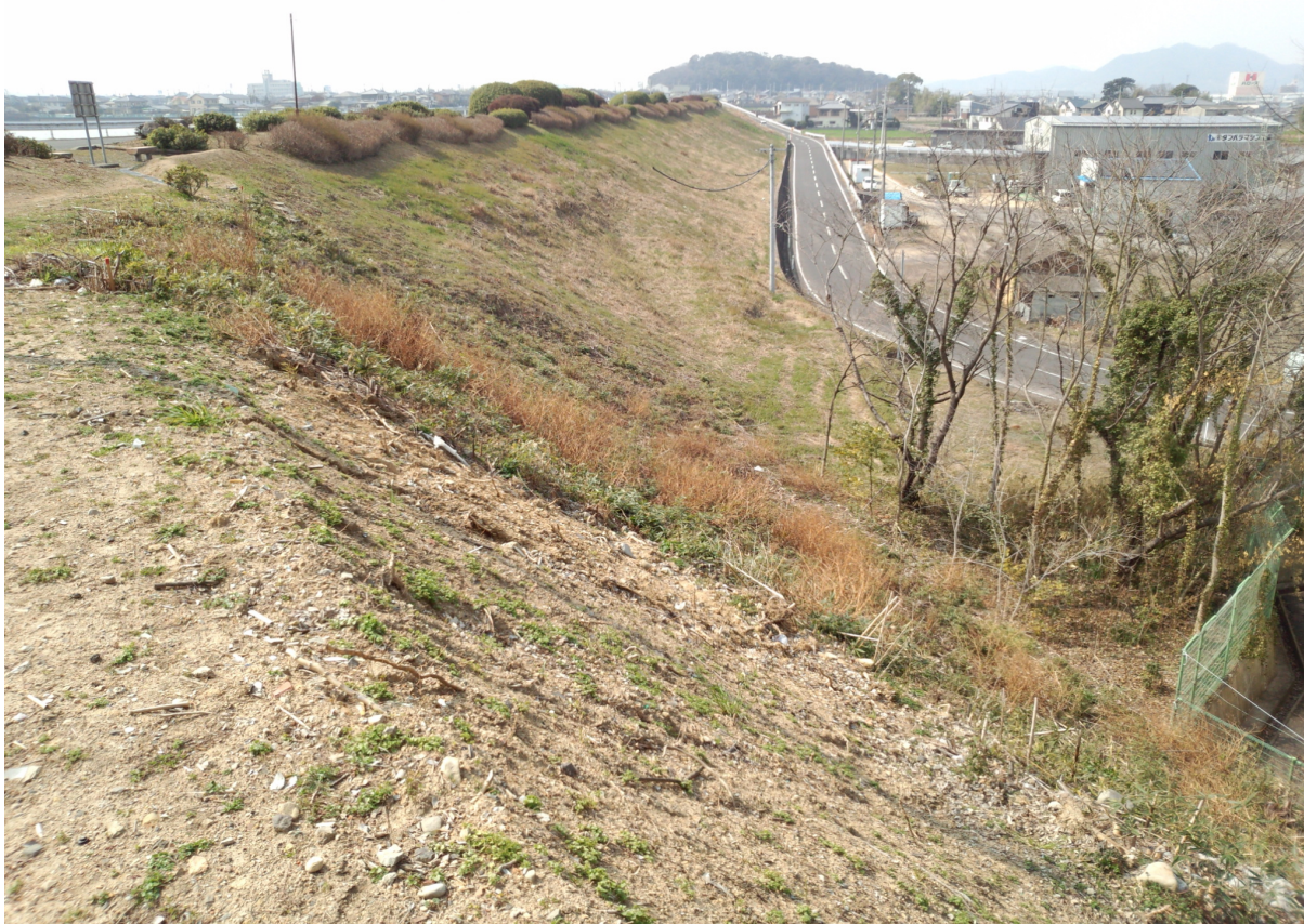
Photo 3.1 Surroundings of Heike (photographed from the eastern end to the west at the top of the embankment)
